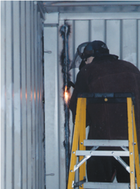
Photo 2.21 / Cutting out a front corner post using an oxygen-acetylene torch. Note that the torch is being pointed in the direction of travel, to preheat the metal to be cut.
