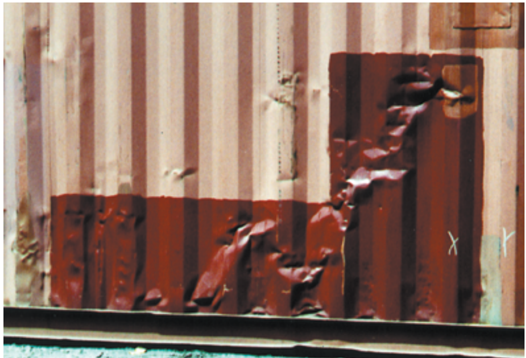
Photo 6.4 / Example of poor panel straightening. The damaged area has been painted, but no attempt has been made to straighten the dents.
