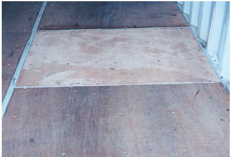
Photo 9.8 (to right) / New plywood panel section in place with sealant applied along edges
