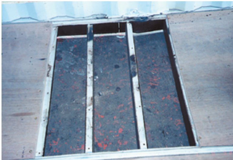
Photo 9.4 (to left) / Removal of plywood panel section, showing joint lying above center line of crossmember flanges
