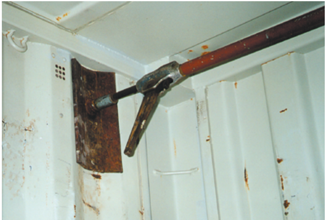
Photo 2.4 / Using a jack with a backing plate to straighten a side panel
