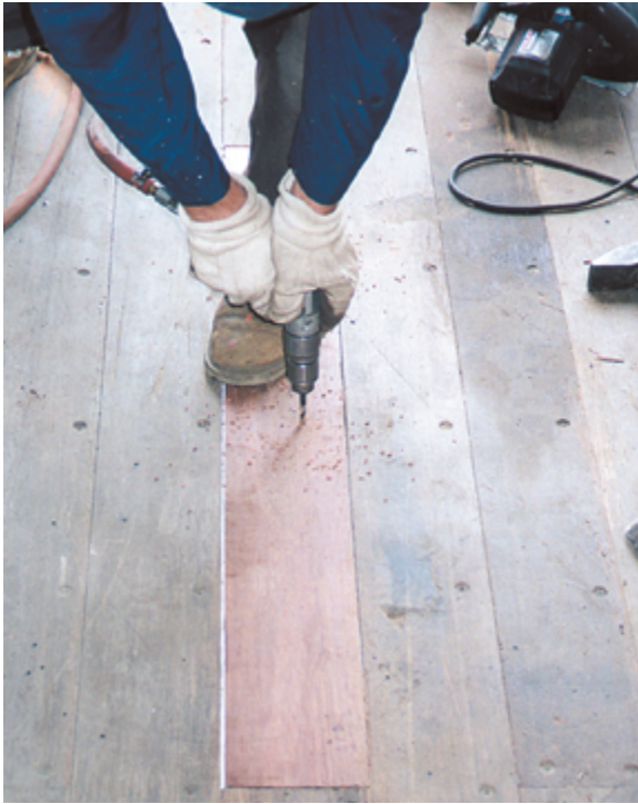
Photo 9.9 (to left) / Drilling new screw holes aligning with line of screws in adjacent planks, following the original floor screw pattern
