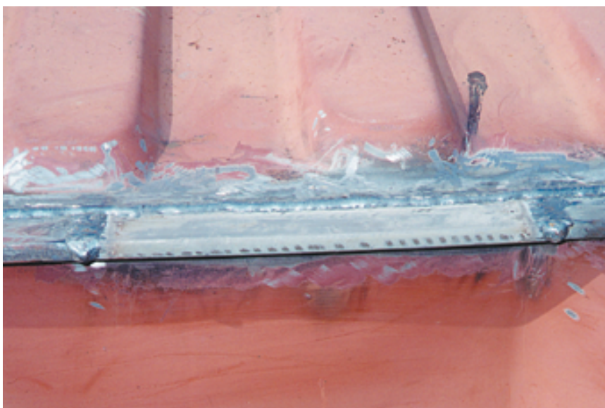
Photo 5.6 (to right) / Completed welding of flat-bar top side rail section. A portion of the welds between the section and the original rail has been ground down to permit proper reattachment of the roof sheet.
